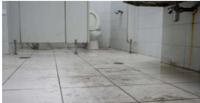
Floor mess with water spill
